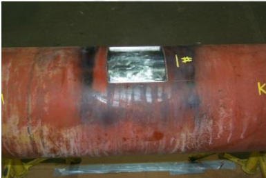
Defect – 6.5" x 6.5" x .300" Deep
